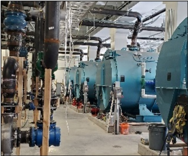
The RWHTF Biogas Utilization Project (PAR 1395), led by Metro Project Manager A.D. Norford, will commission the Boiler Mechanical Facility in the third quarter of 2026, a critical early milestone necessary to maintain essential process heating after CHP decommissioning and prepare the site for Biogas Upgrading Facility construction.
