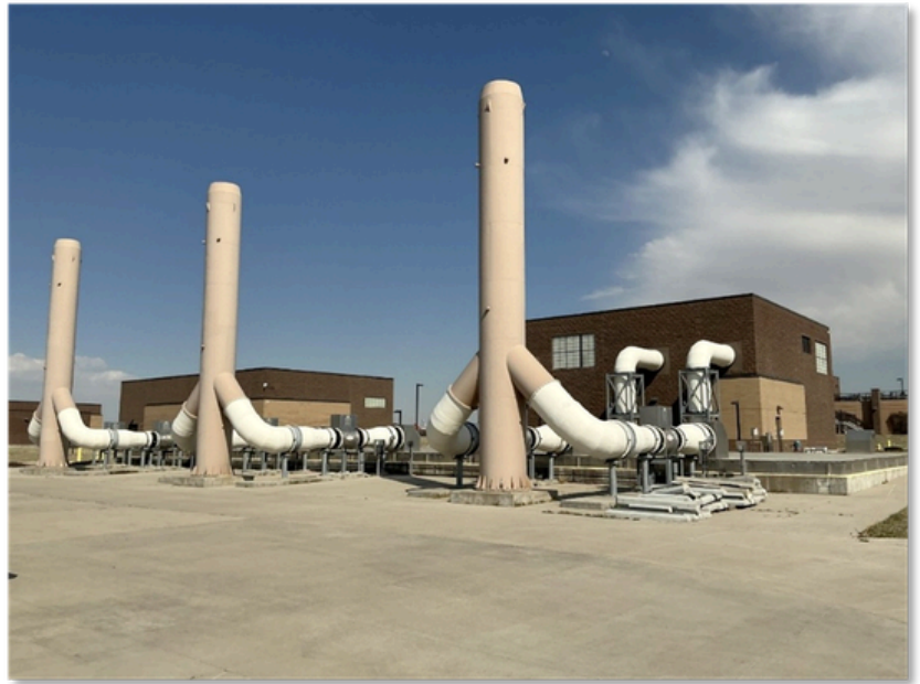
Figure 6 – Odor control technology at NTP
