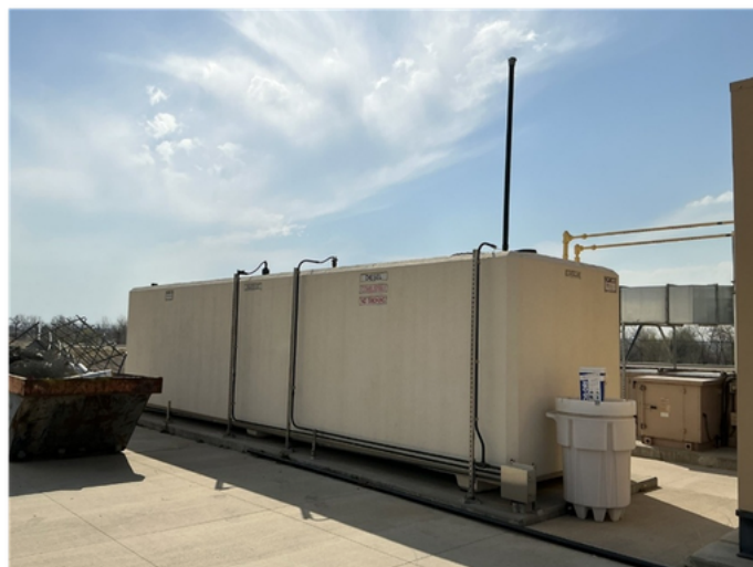
Figure 2 – Northern Treatment Plant emergency generator, a 12,000-gallon auxiliary diesel tank
