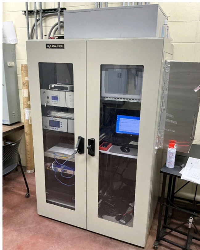
Figure 4 – analyzers monitoring H 2 S gas concentration in the anaerobic digesters at RWHTF
