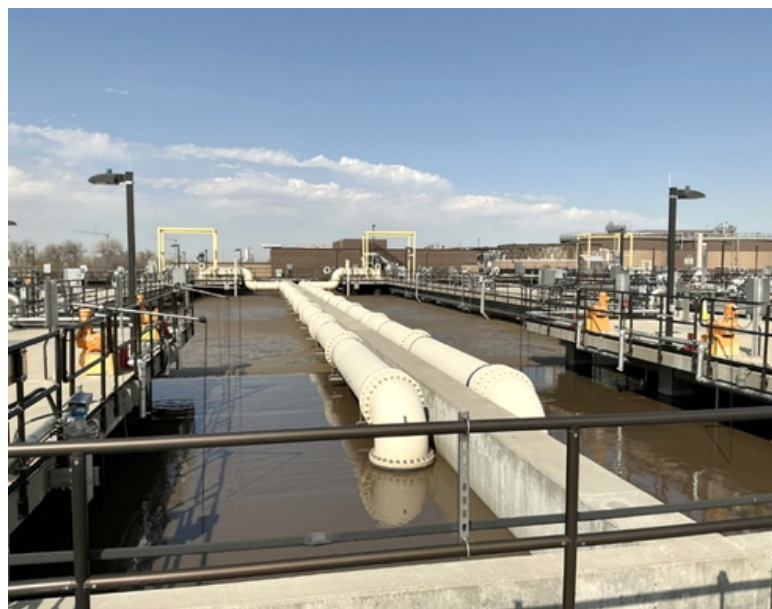
Figure 5 – Fugitive VOC emissions may occur during the wastewater treatment process
