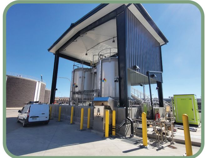
New PAA dosing bins at RWHTF.
