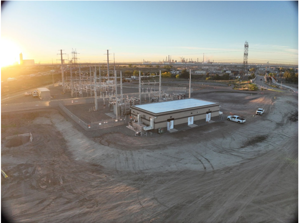
The new electrical transmission service substation at Robert W. Hite Treatment Facility.
