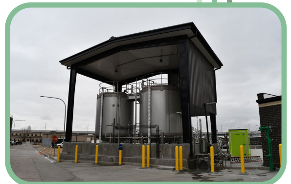
The new peracetic acid disinfection system
