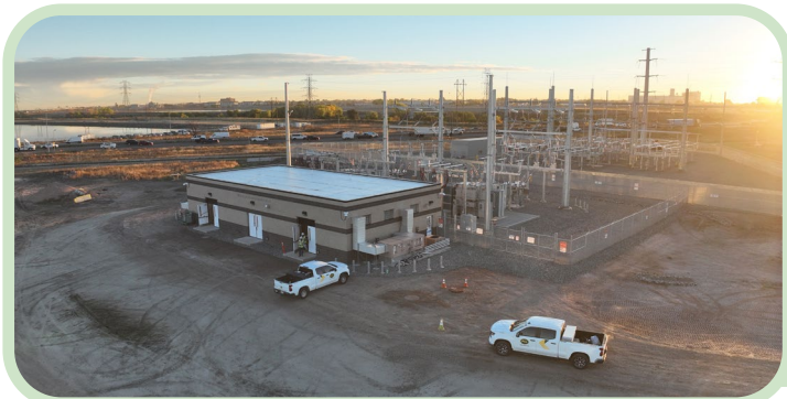
Electrical transmission service substation
