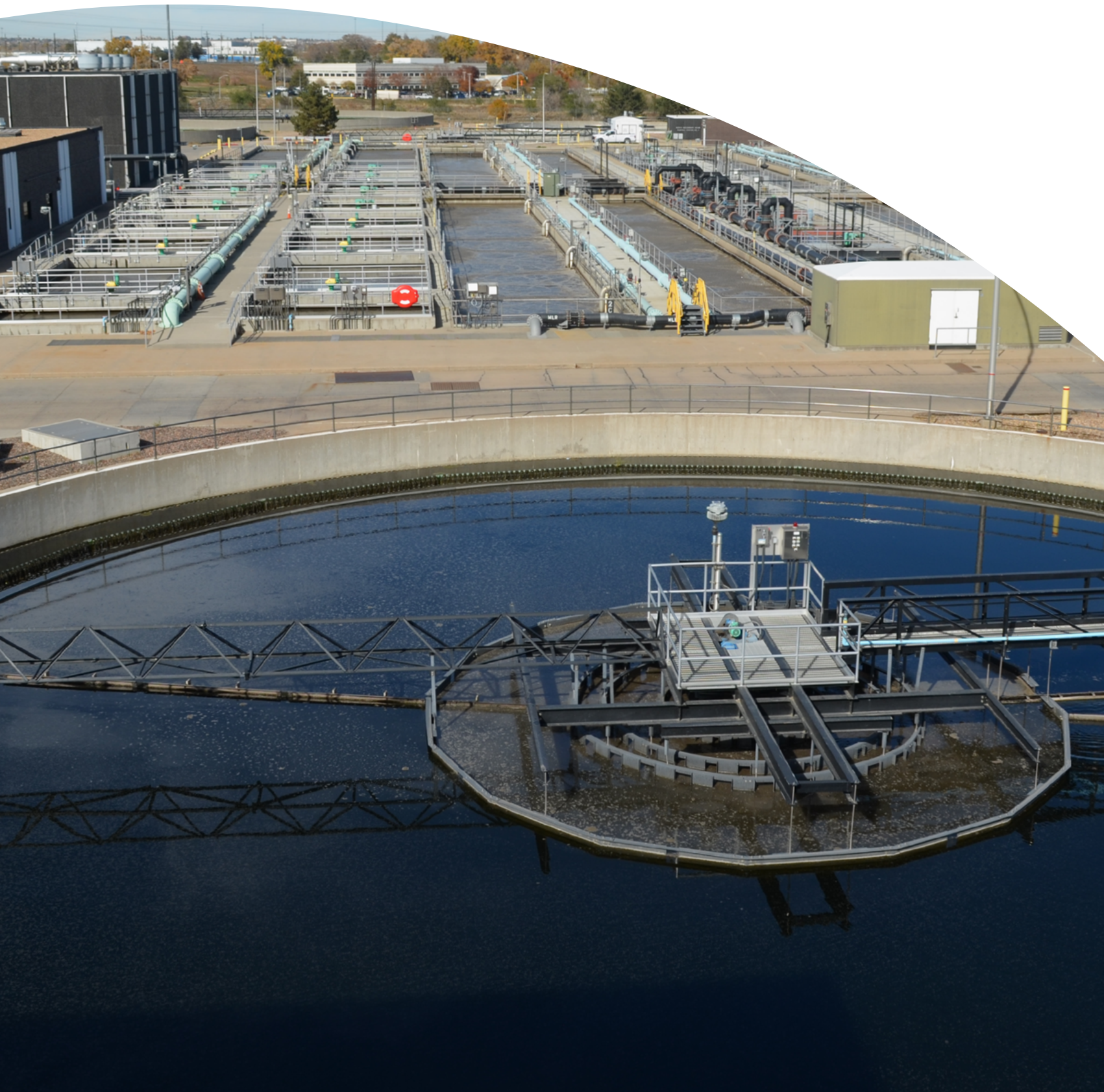
RWHTF North Plant clarifier and aeration basins.
