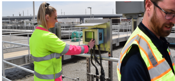
Cassie Caley, In-Line Instrument Specialist II, checking an instrument panel in the RWHTF South Plant.
