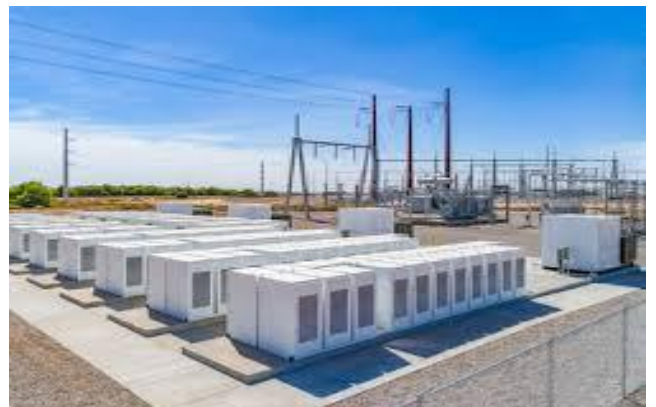
Figure 3 – Battery storage facility
