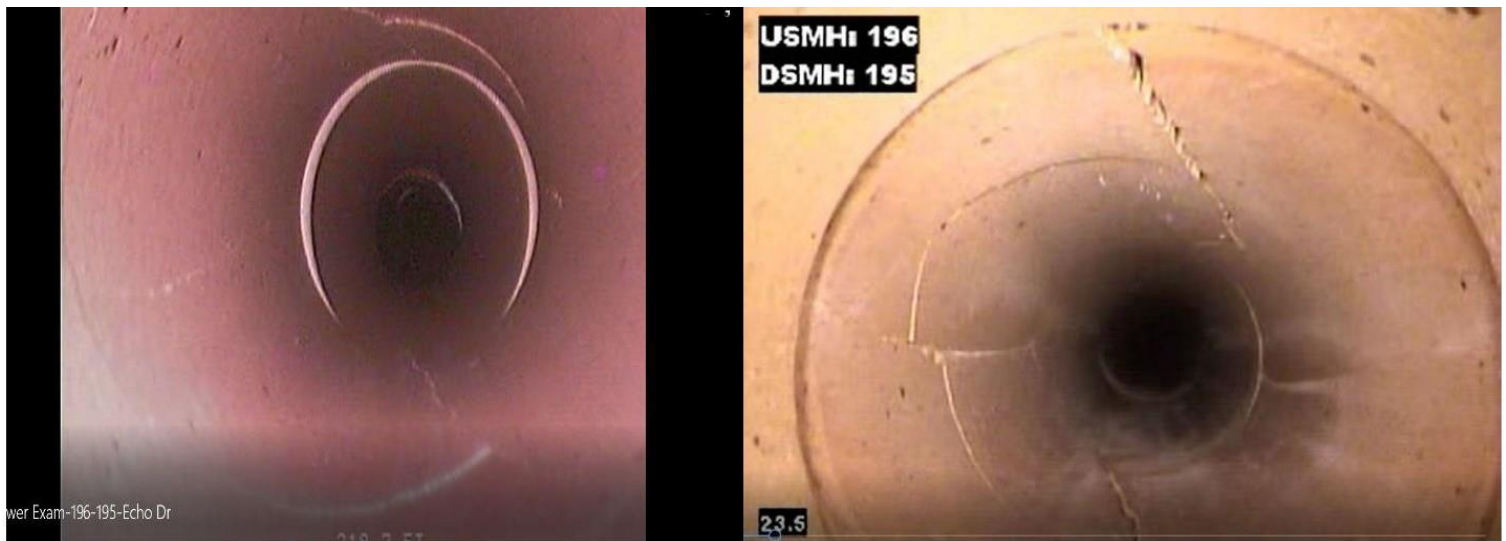
2013 Figure 3 - Photographic Comparison of a Cracked Pipe from a Rate of Deterioration Analysis
