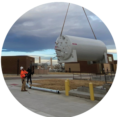
Contractors remove NTP's liquid oxygen tank as part of the post-aeration decommissioning process.
