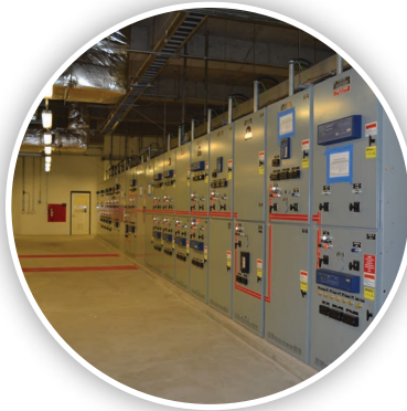
South Secondary electrical switchgear.
