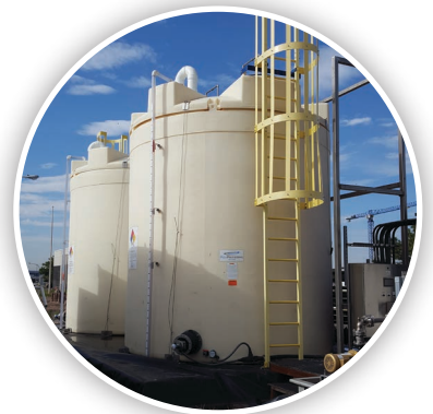
PAA tanks on the Robert W. Hite Treatment Facility.
