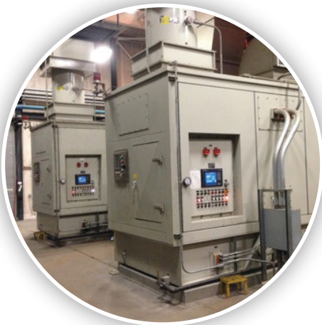
Combustion turbines for combined heat and power system.
