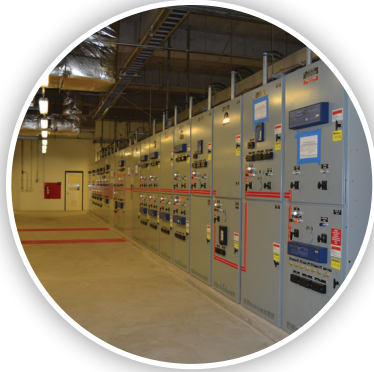
South Secondary electrical switchgear.
