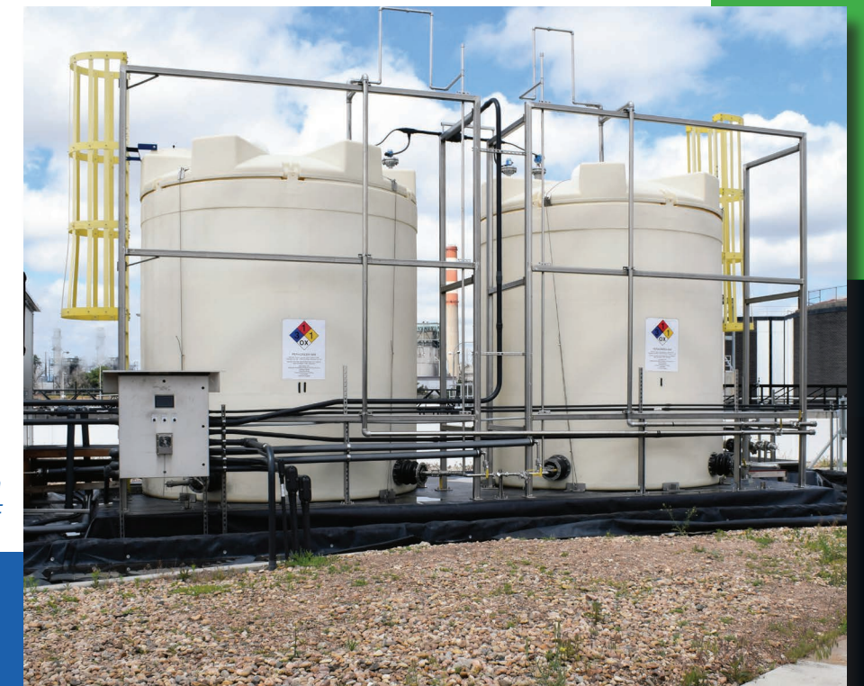
PAA Dosing System at the RWHTF
