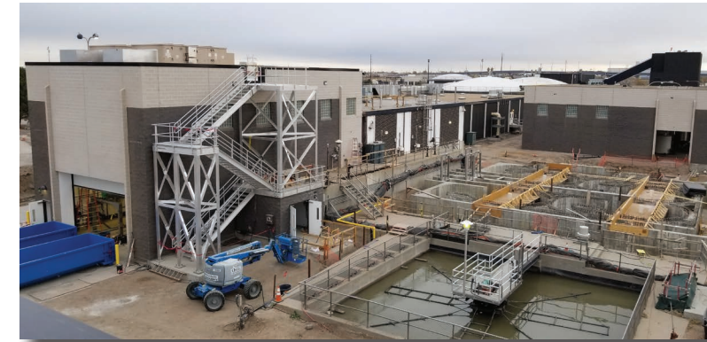
Above and opposite page: Construction for South Headworks and Grease Processing Improvements Project
